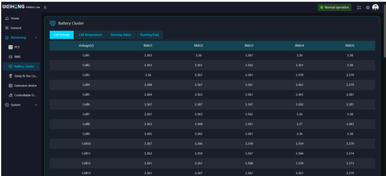
Figure 6-6 Operation Monitoring – Battery Cluster Screen
